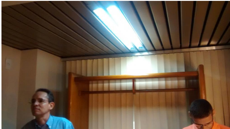
Figure 2.7: Fluorescent light at a Dressing Room.
