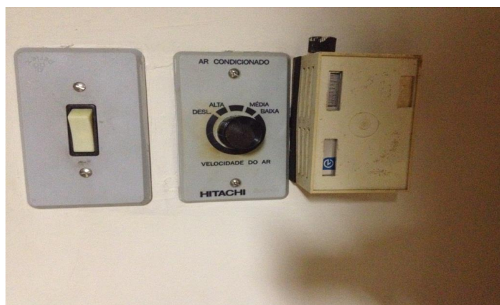
Figure 2.8: Control to turn in/off the air conditioner.
